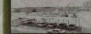
Resources Mobilisation of resources for the construction of the 39-storey building that took five years to complete.
